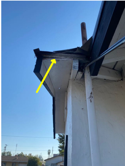
Drip edge missing on north side of home
