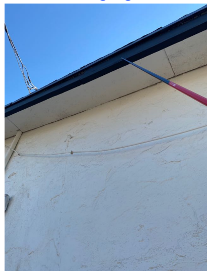
Exposed roof sheathing on west side of home
