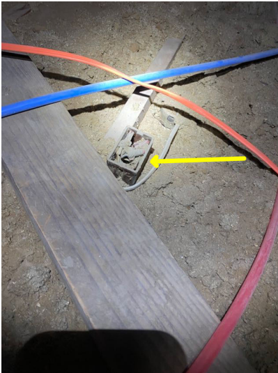
Open electrical box
