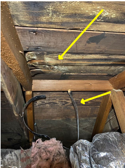
Damaged roof sheathing
