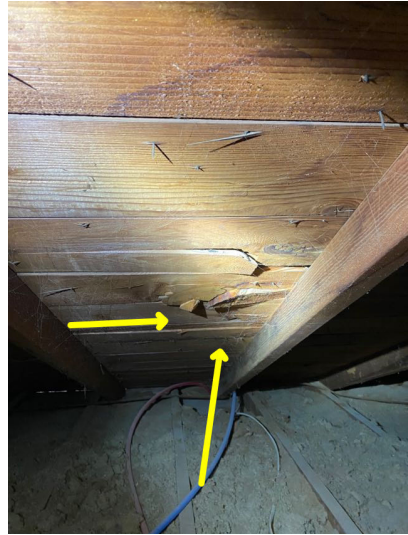
Damaged roof sheathing
