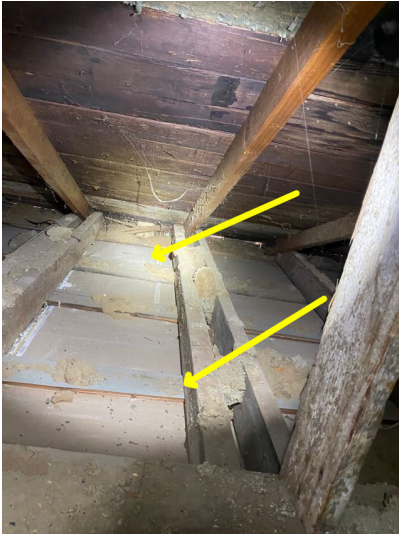
Missing insulation over living room
