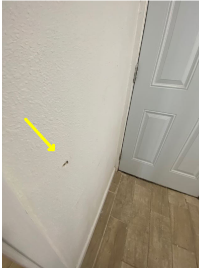
Back entrance door is missing door stop.
