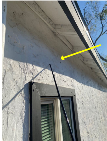
Stucco appears to be separating or bulging.
